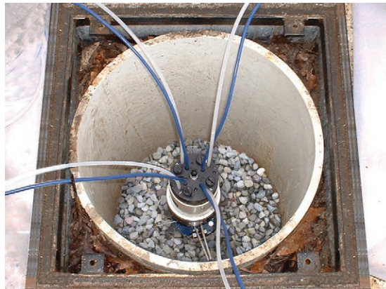
Figure 9-1 Tubing Organized Around the Wellhead
