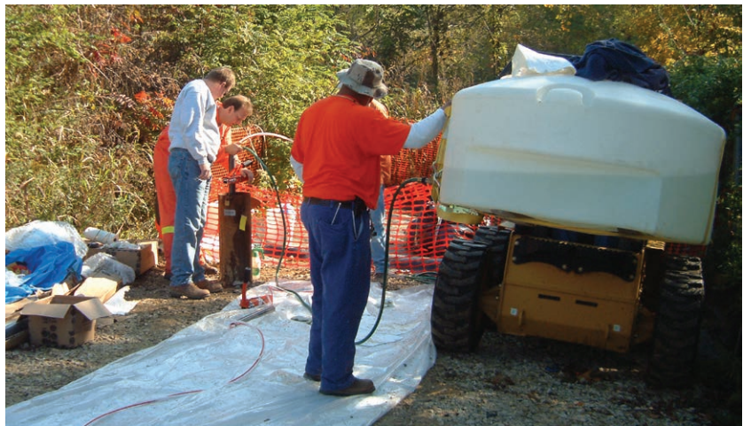
Figure 8-1 Adding Water to the System
