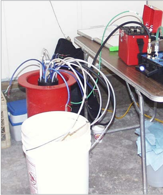
Four Waterloo Systems were installed to monitor a chlorinated compound release. Systems were installed at depths ranging from 131 m – 229 m (430 ft – 750 ft), with most monitoring 7 zones. The Ports were constructed with both Double Valve Pumps and Vibrating Wire Transducers.
